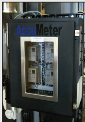
Motor Drive Panel
