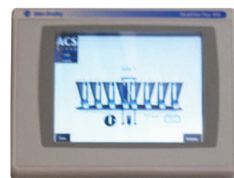
Allen-Bradley Control System Interface
